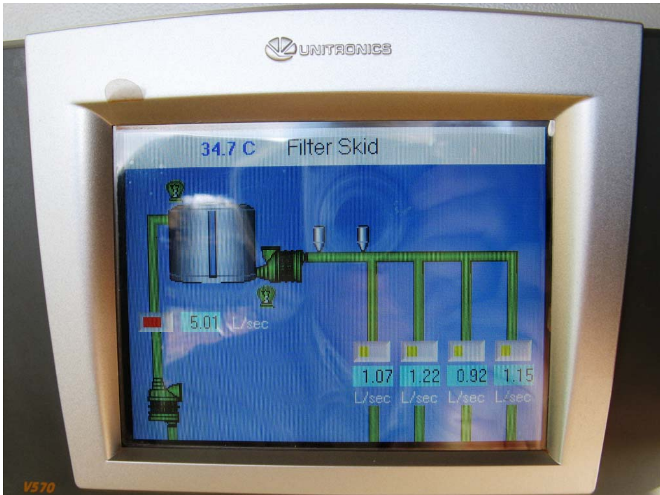
Solution flow rates in Litres/second as shown in well house control panel for extractor well (at left) and four injector wells (at right).
