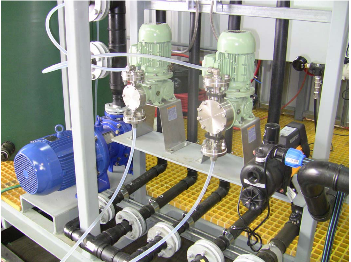
Figure 2 : Detail of acid and peroxide dosing pumps, completed well house unit
