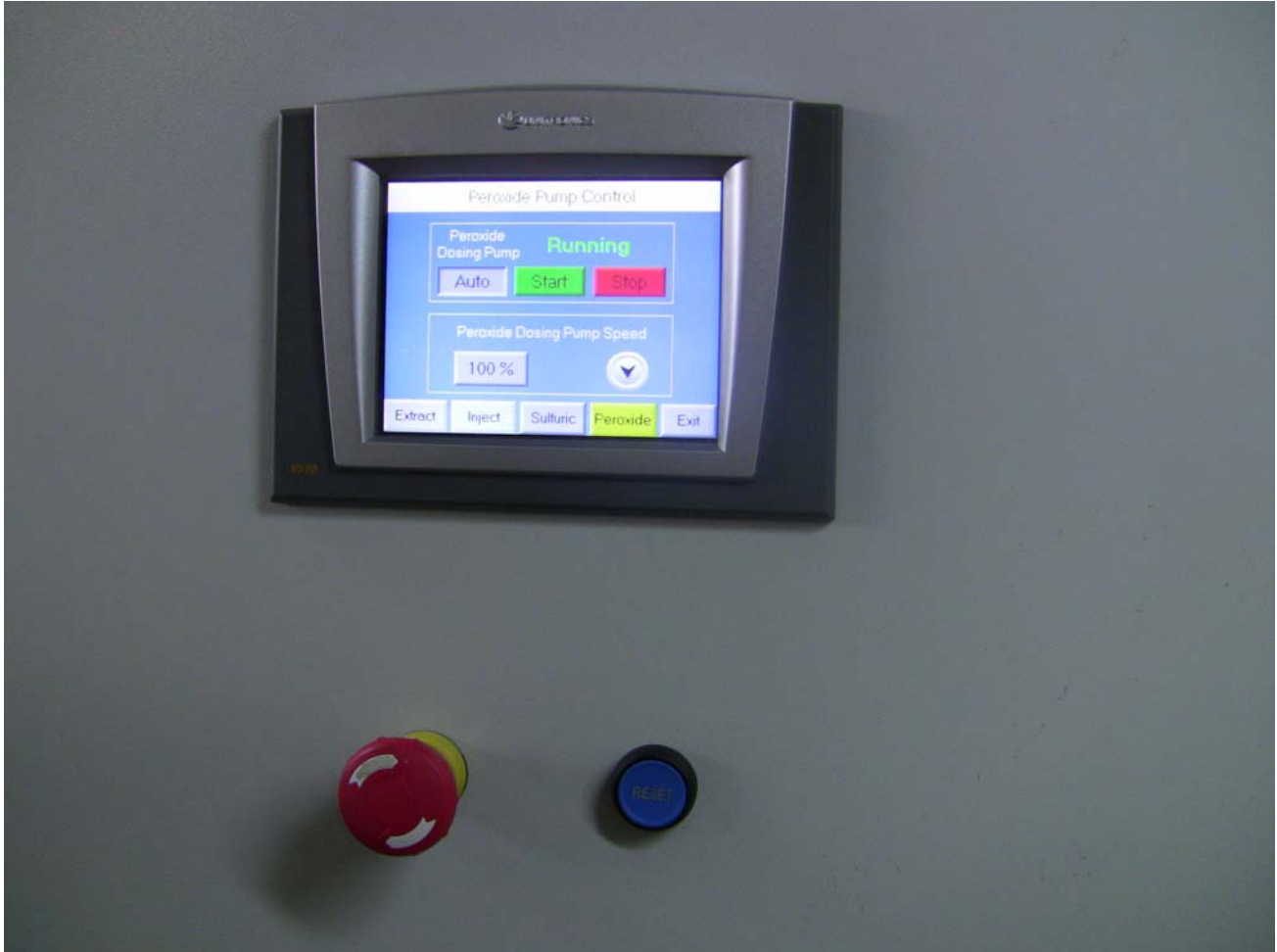
Figure 3 : Automated dosing of acid and peroxide in circulating solutions
